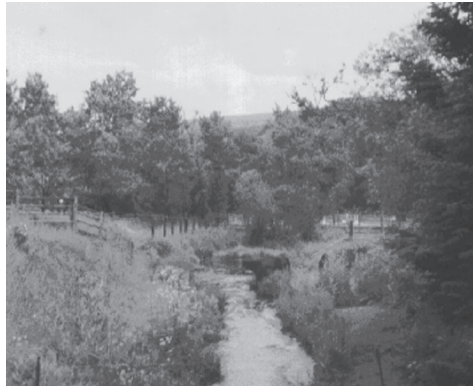
Figure 421312-1. Horse-broken-down stream bank
